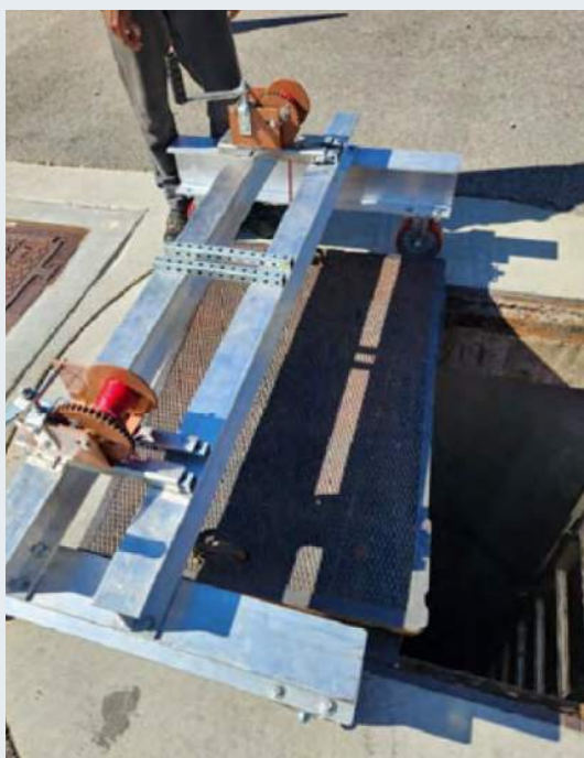
NV5 designed and manufactured a special tool to remove, secure and replace the gate shaft access lid (approx. 500 lbs each) so that proper access could occur.
