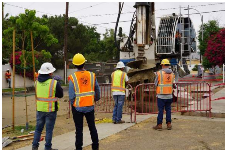
Geosyntec designed and substantially constructed over $17M of green stormwater infrastructure, including over 60 drywells, for the City of LA in just 18 months. Geosyntec also provided 1 year of performance monitoring and maintenance for the built green stormwater infrastructure.
