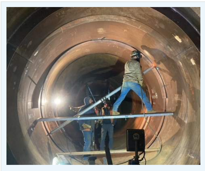
Buntich's Etiwanda Pipeline North Liner Repair Project in Rancho Cucamonga, California for Metropolitan Water District.
