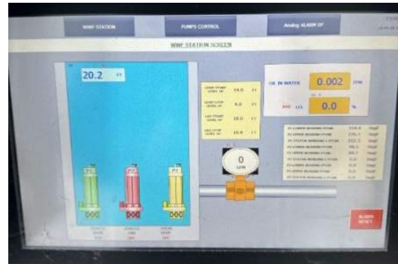
Geosyntec investigated, troubleshoot, and updated PLC programming to restore automation and partial capacity for a 50-cfs stormwater pump station at LAX Airport.
