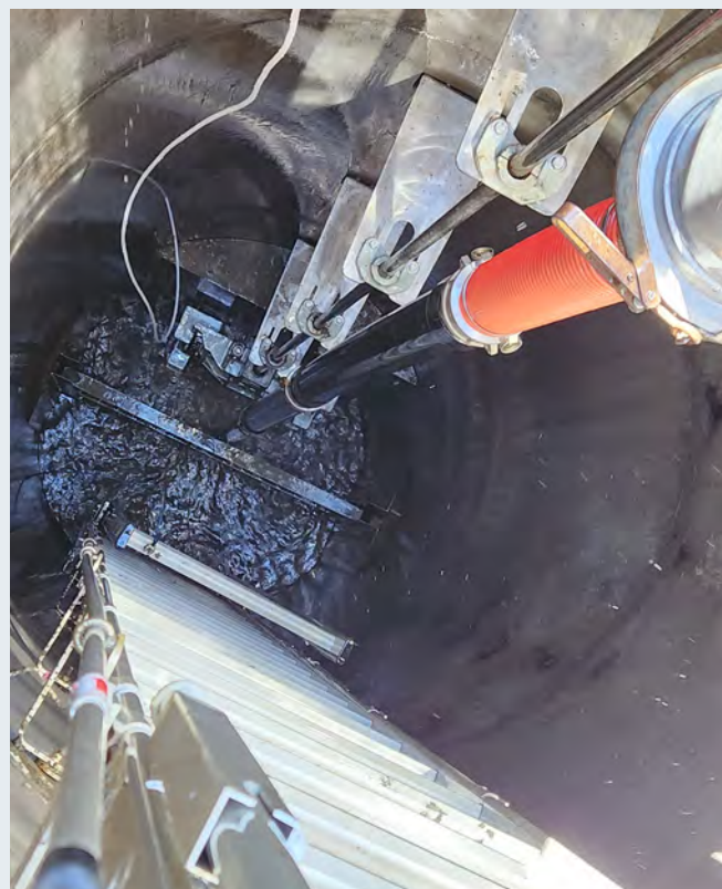
Vector/hydrojet and maintenance service for the Gates Canyon Motor Operated Slide Gate Pre-storm Season Service. Trash rack and slide gate components were cleaned and shaft and spline and gate features were lubricated per specification.
