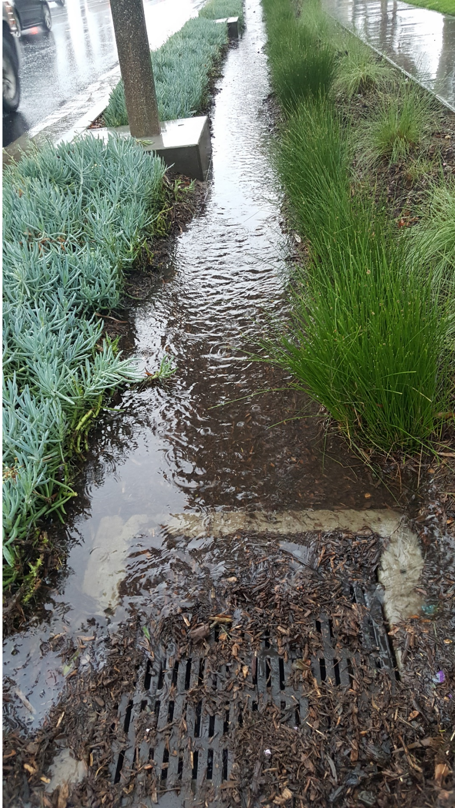
Figure B-4. Outflow from the Downey Bioswale and the Outflow Sampling Point during the January 12 Event.
