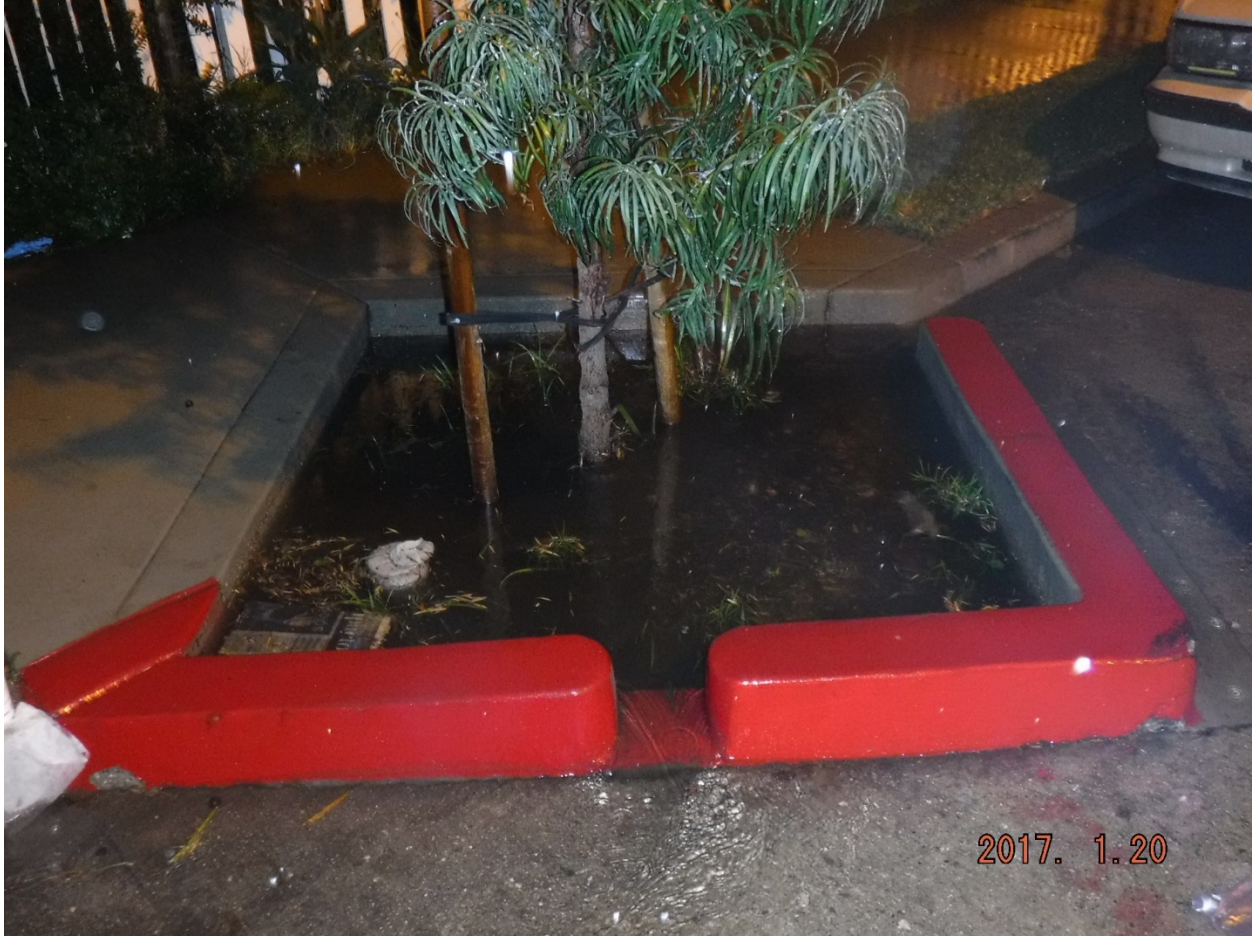
Figure B-18. Outflow from the Whitter Tree Well at 7751 Milton Ave. during the January 19 Event.
