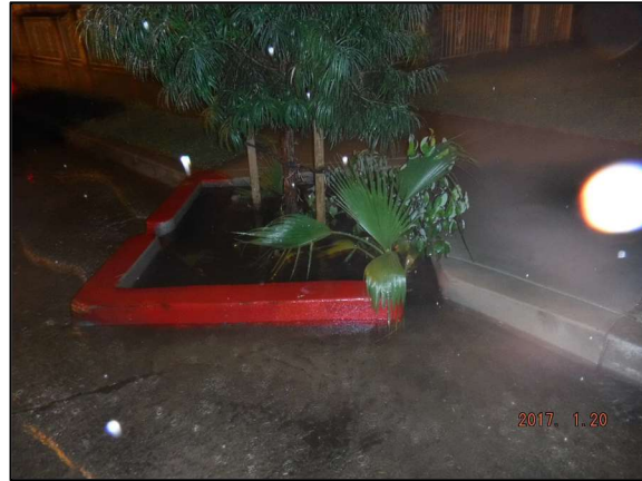
Bioretention Tree Well -7913 Milton Avenue (January 19 th Storm Event)
