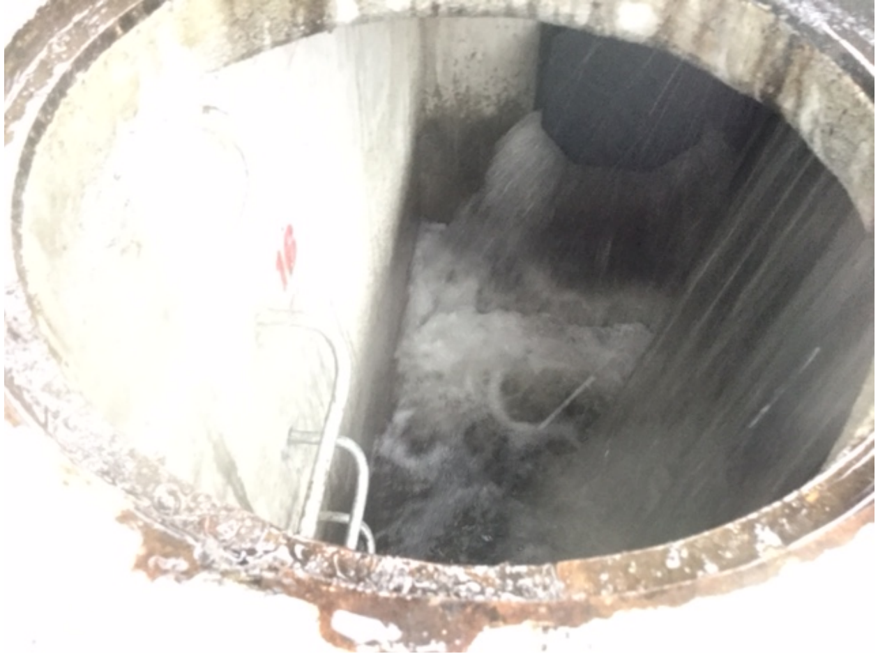
Figure B-8. Outflow Sampling Point from the Downey Bioswale during the February 17 Event.
